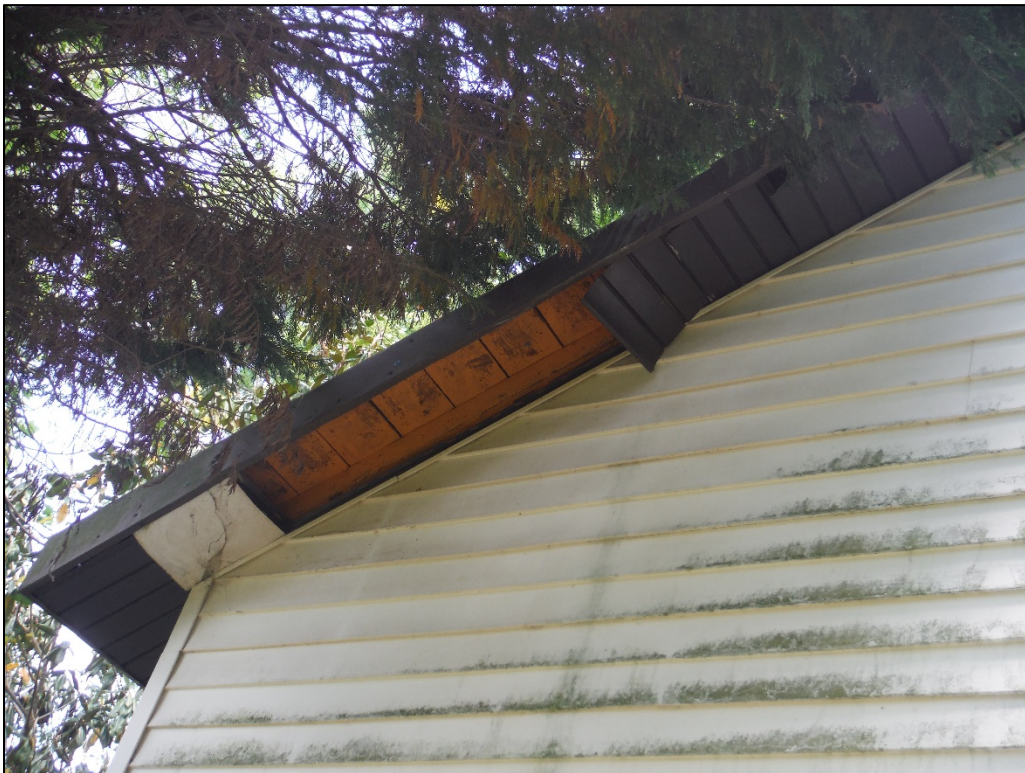
Figure 12. View of the (former) Mooresboro School, roof construction on west elevation, facing east.
