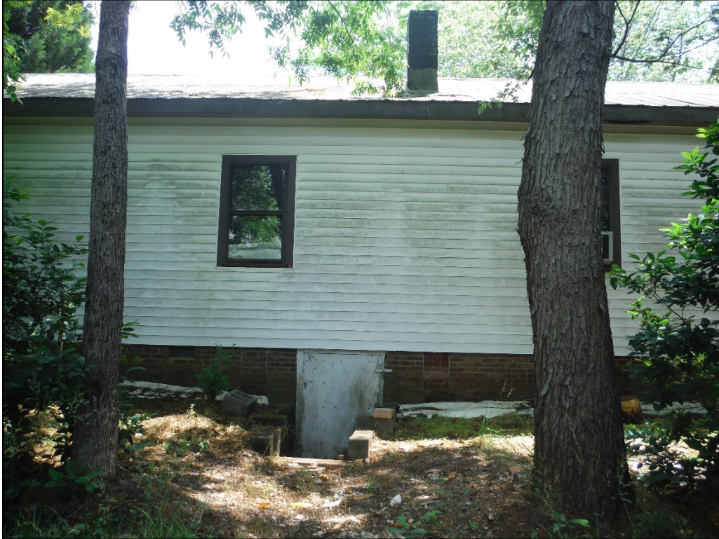
Figure 7. View of the (former) Mooresboro School, foundation and basement door, facing south.
